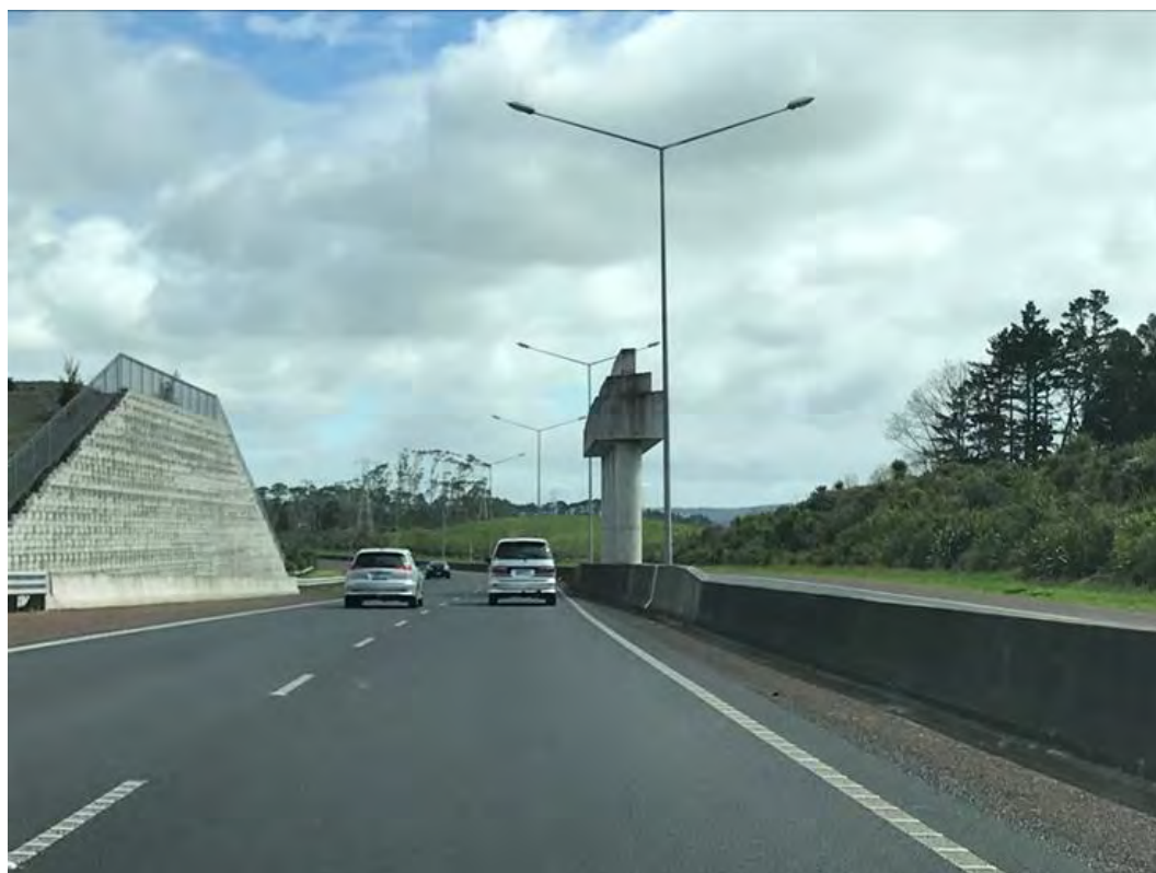
Figure 3: Pillars located on State Highway 16 to support the future Northside Drive extension
